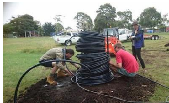
The beginnings of compost shower for the Good Life Permaculture Design Course.
